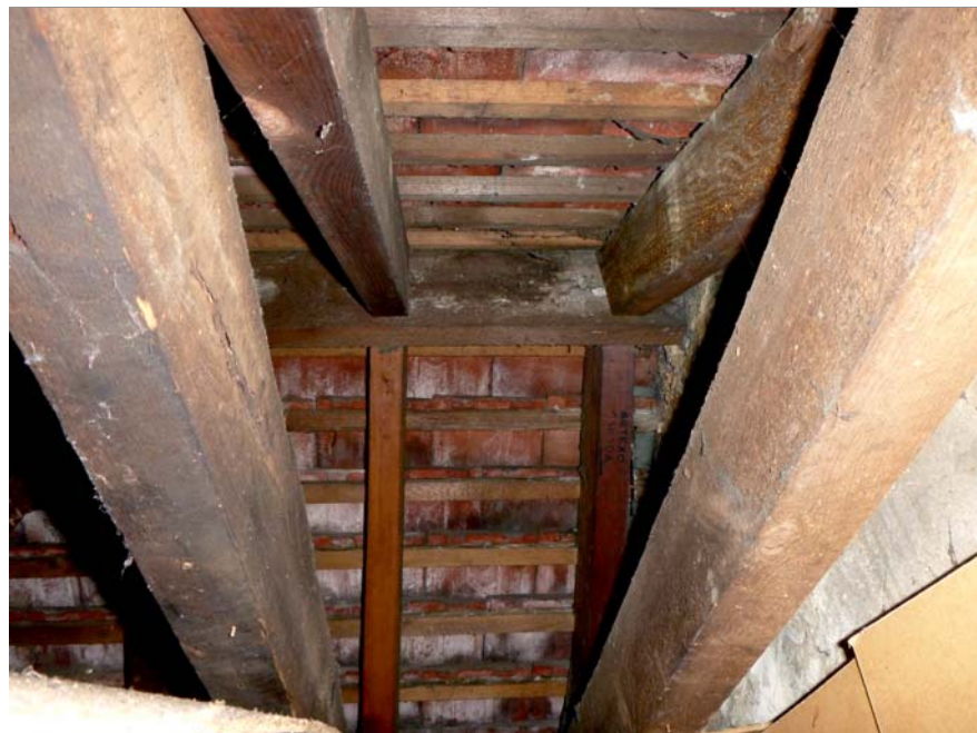
Photograph 3: Showing the unlined attic space, exposing the undersides of the roof tiles.
